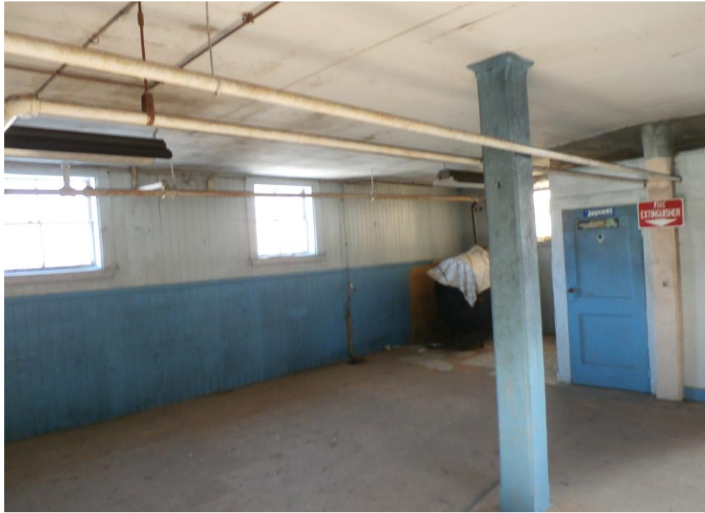
Figure 4: Basement Oil Tank & Furnace Enclosure
